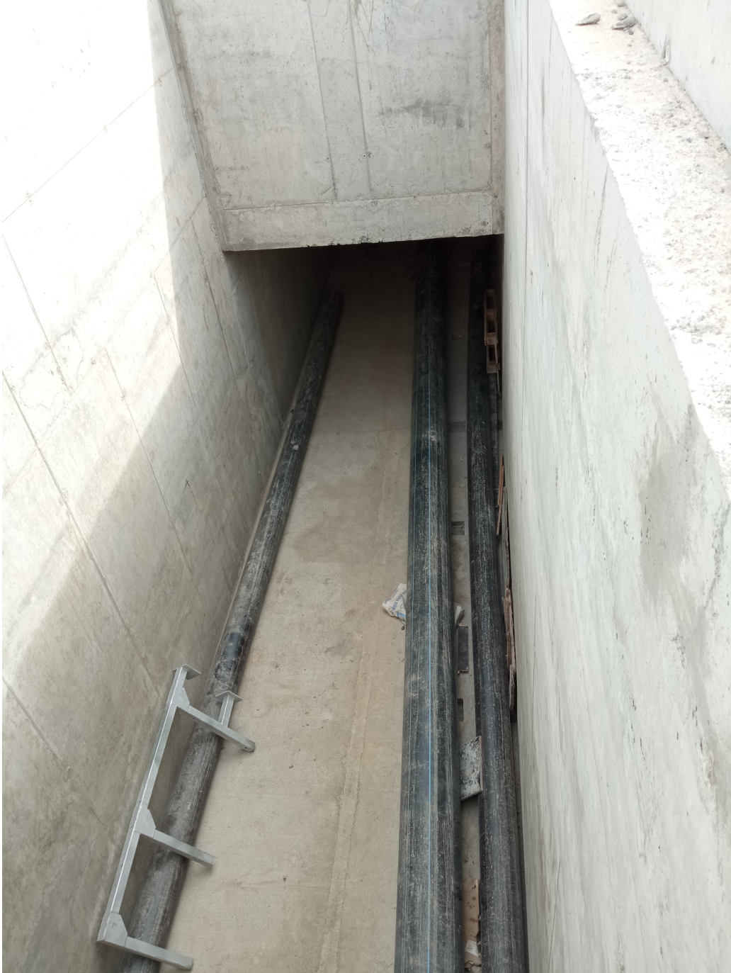
The Tunnels that will house all piping and cabling
