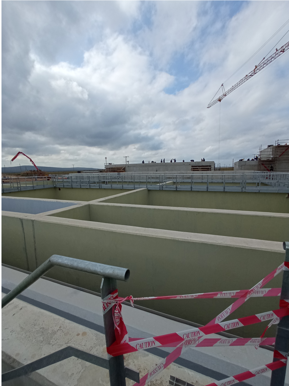
Wastewater reclamation facility
